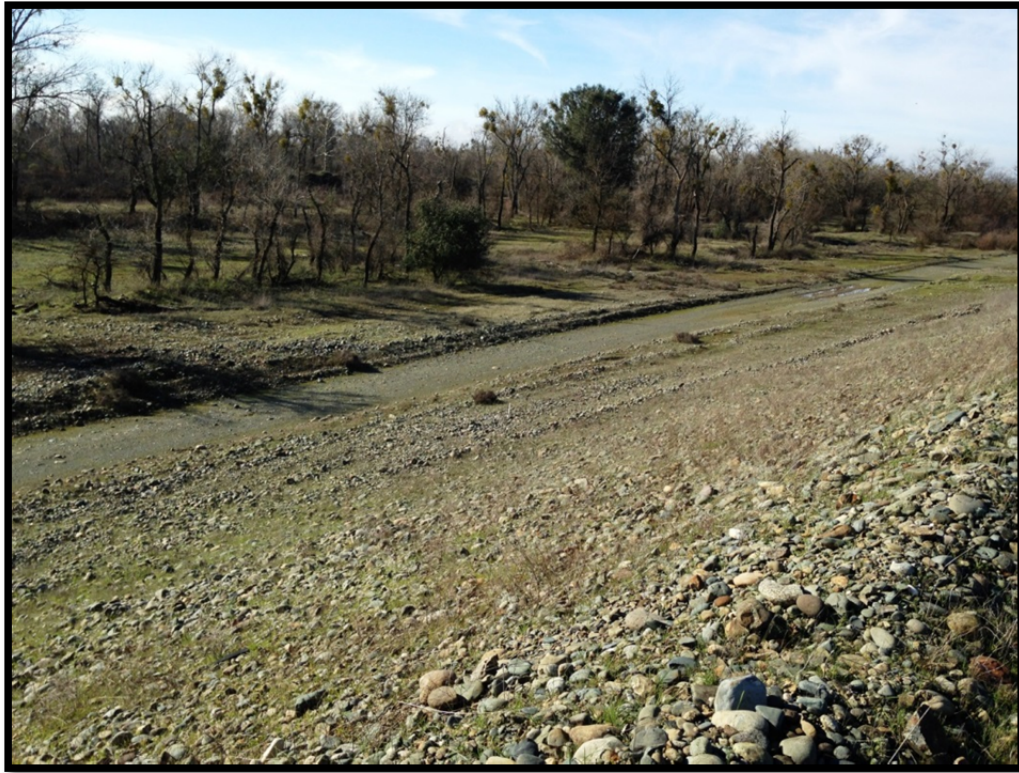
Figure 3. Site 2 - Inlet Weir Location looking Downstream at the OWA Side of the Existing Levee
